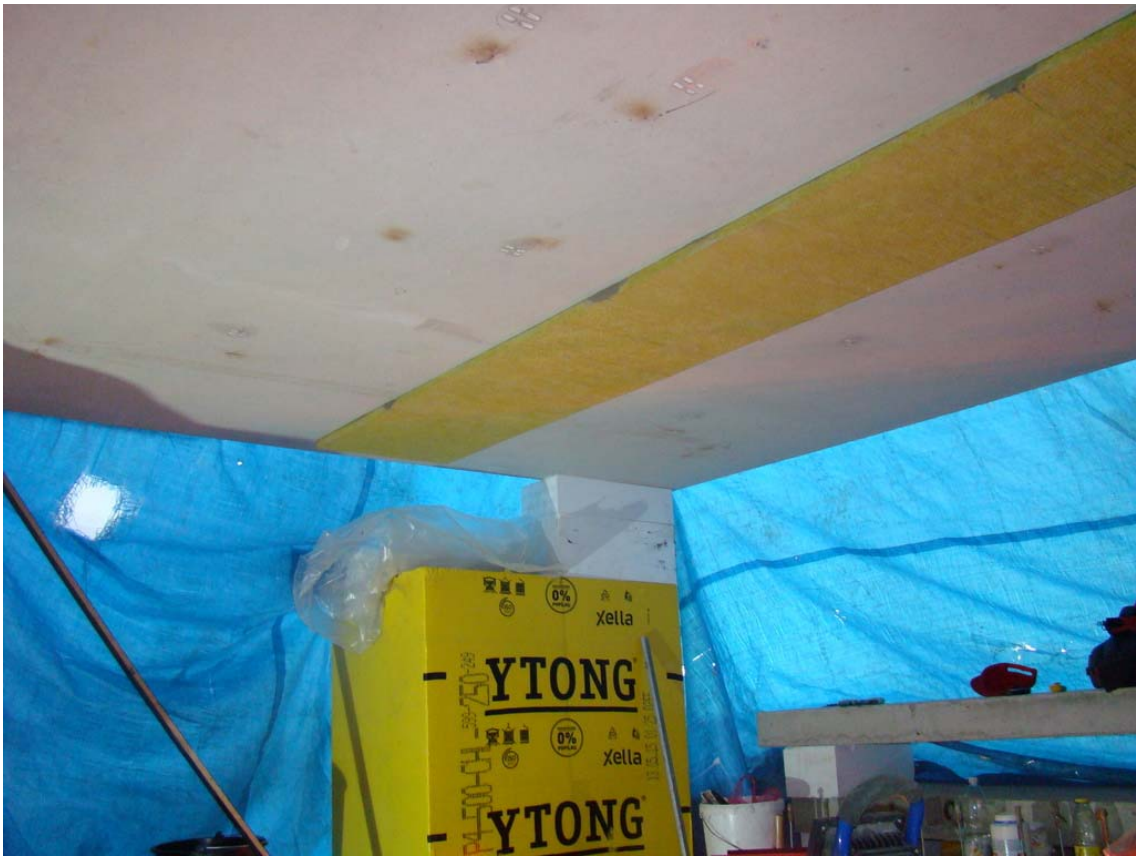
Installation of the first row of slabs - inspect the straightness of the row
